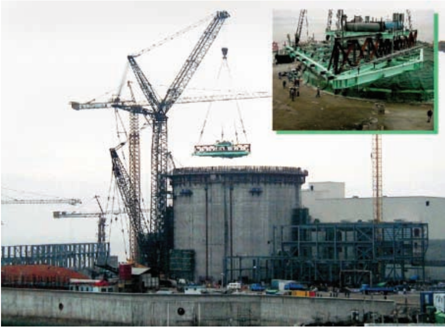
FIG. 236. Qinshan site: VHL crane lifting dousing system module through open top of reactor building (June 2001).
