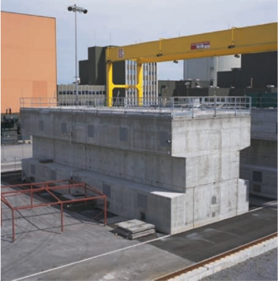
FIG. 137. The MACSTOR facility at the Gentilly 2 reactor.
